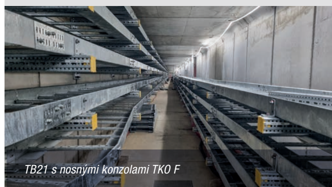
siFramo Supports v budove Tokamak
